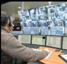
Command and Control Rooms
