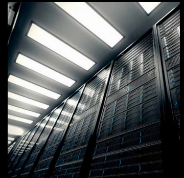
Data Center and IT Infrastructure
