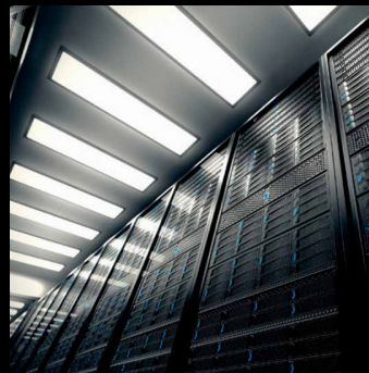
Redundant and Remote Networking
